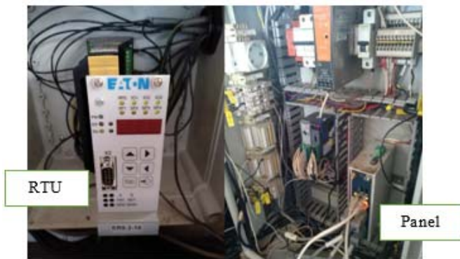
Fig. 9. RTU and Instrument Panel
